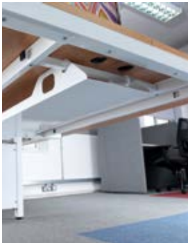
Cable tray and vertical risers to ensure complete cable control
